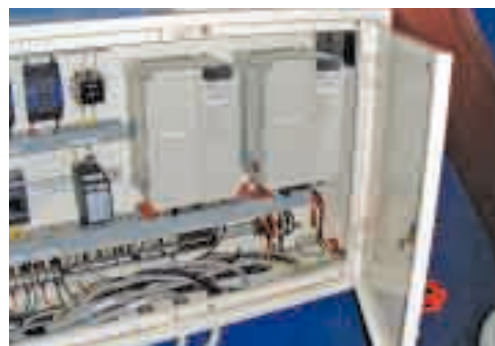
Water pump control panel with inverter installed at the Hamamatsu Plant
